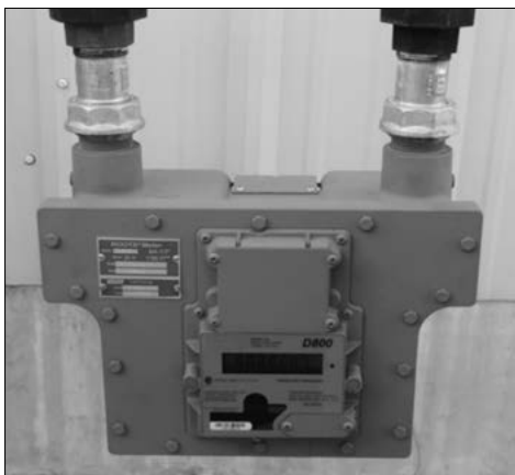
Figure 5.4 -Meter placed in line
