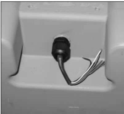
Figure 7.8- Pulse output cable on backside of meter
